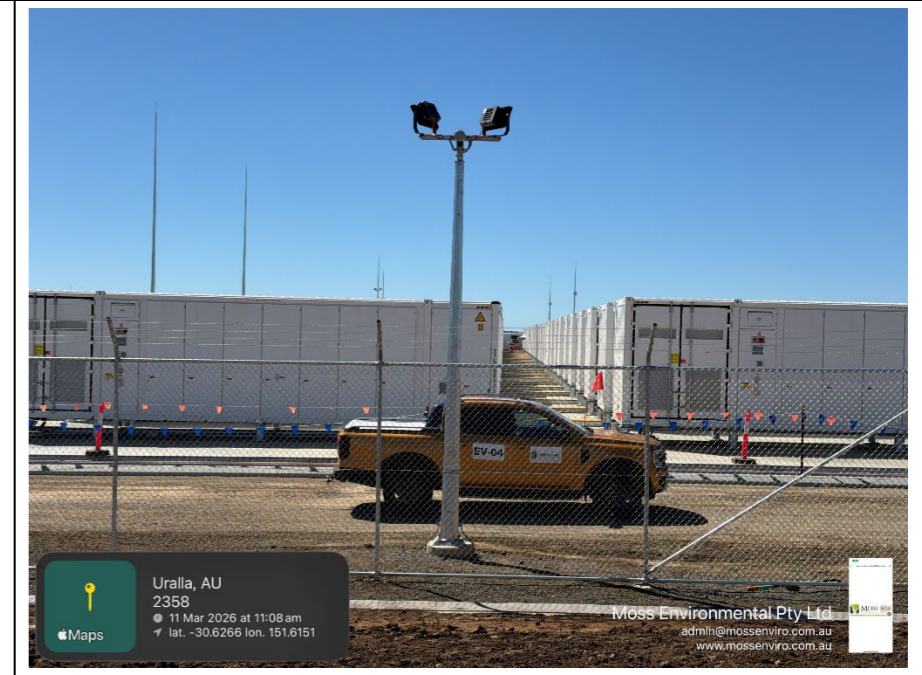
Photo 9 – Lighting at the BESS
