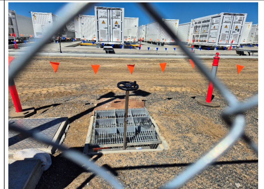
Photo 15 – Valve leading to the sedimentation ponds
