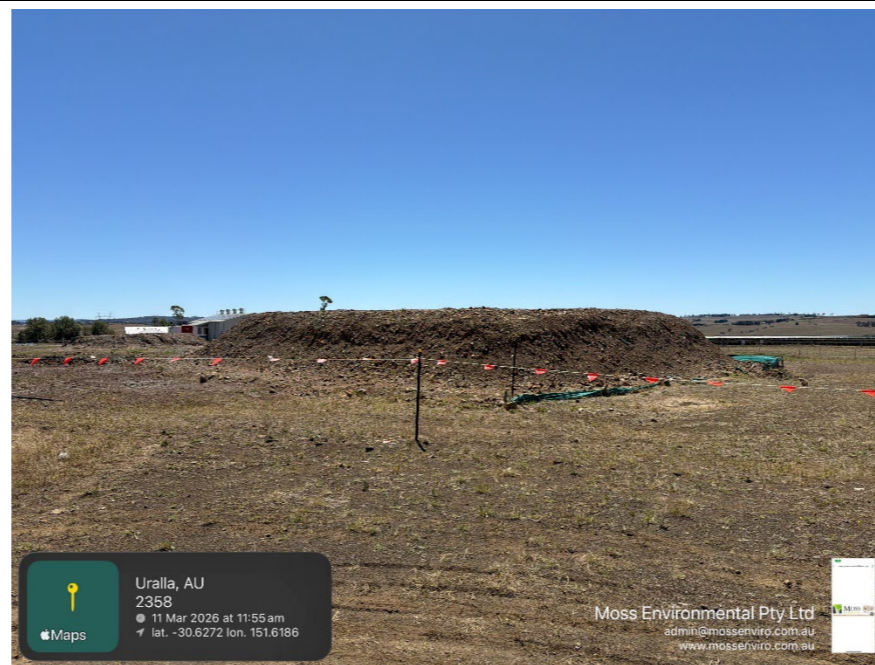
Photo 23 – Silt fence line damaged around the stockpile area
