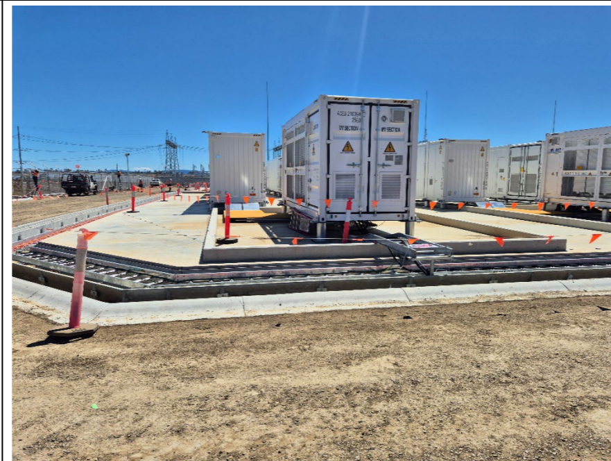
Photo 11 – Colours of the BESS
