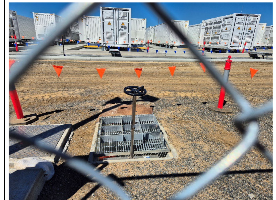
Photo 15 – Valve leading to the sedimentation ponds
