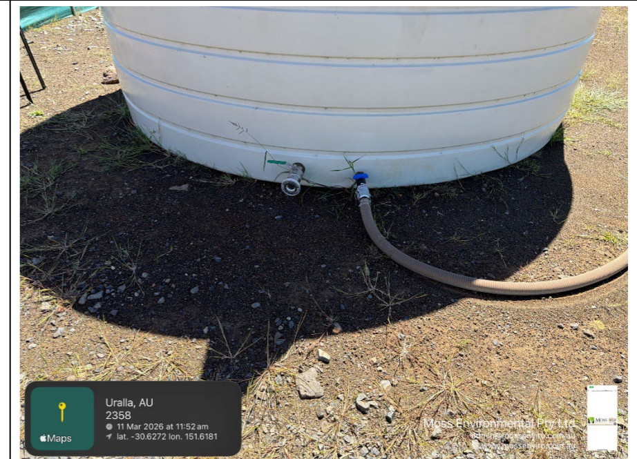
Photo 24 – 20,000 litre water supply tank
