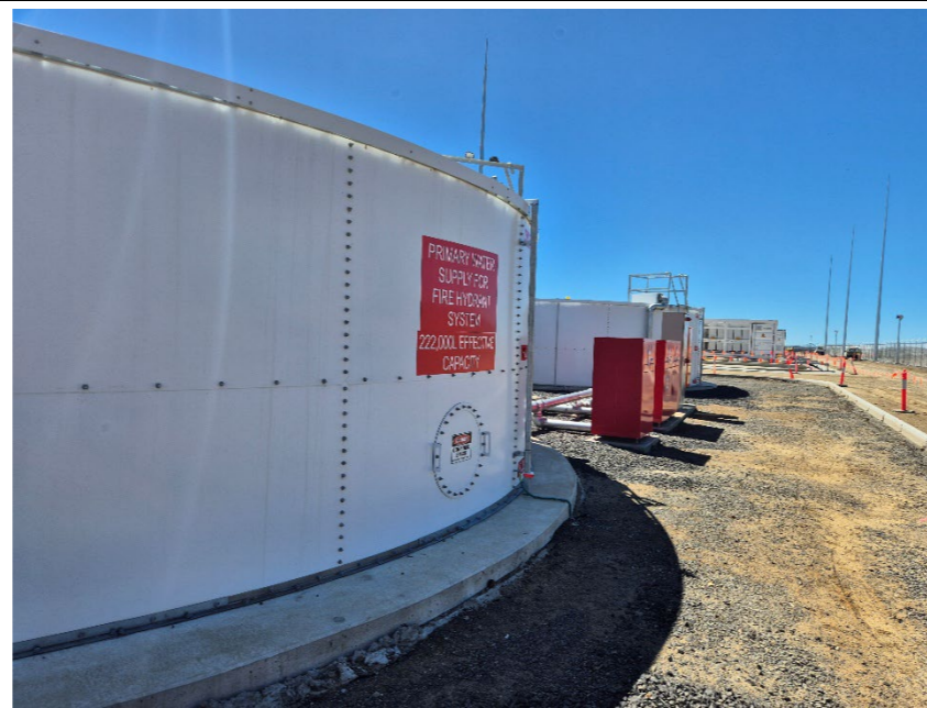
Photo 14 – Fire fighting water tanks
