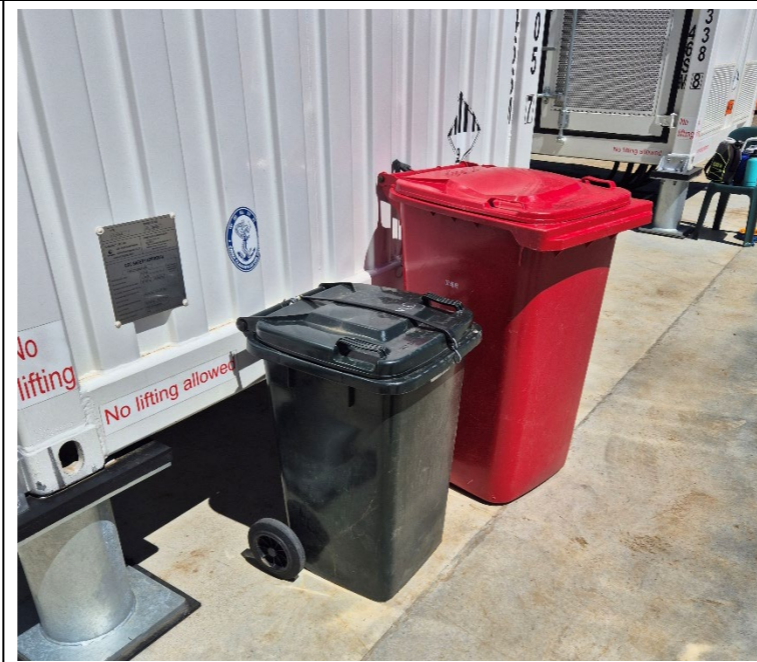
Photo 20 – Unlabelled waste bins in the BESS footprint area
