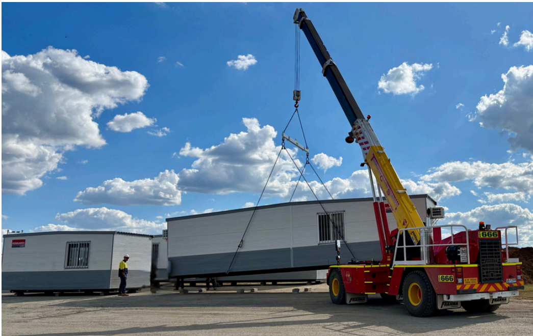
A crane lifts a demountable building into position in April 2025, as the site compound is established. Now the reverse is underway, as the construction compound is demobilised.
